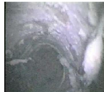
Feed water pipe with sodium hypochlorite
